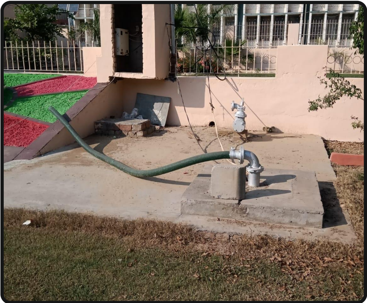
Tubewell in College Campus for Clean Drinking Water
