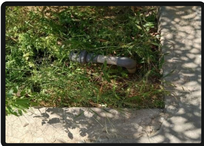
Water supply in park without wastage
