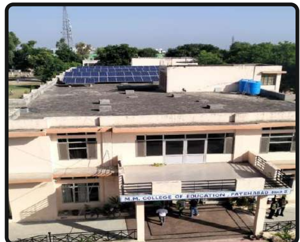
Solar Plant on block -2
