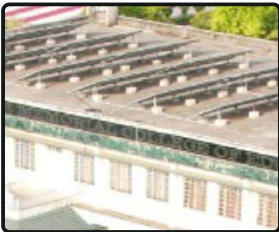
Solar panel on roof of college building Block I
